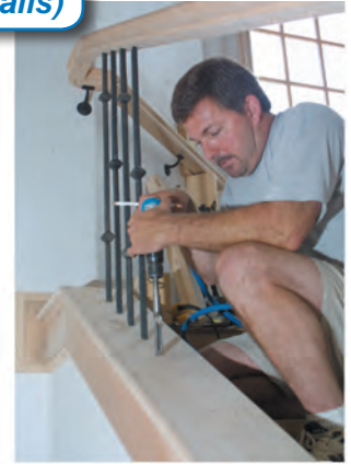
4. Square off bottom hole with air hammer/chisel and mortising bit without the drill inside. (For installation of square balusters without needing shoes)
